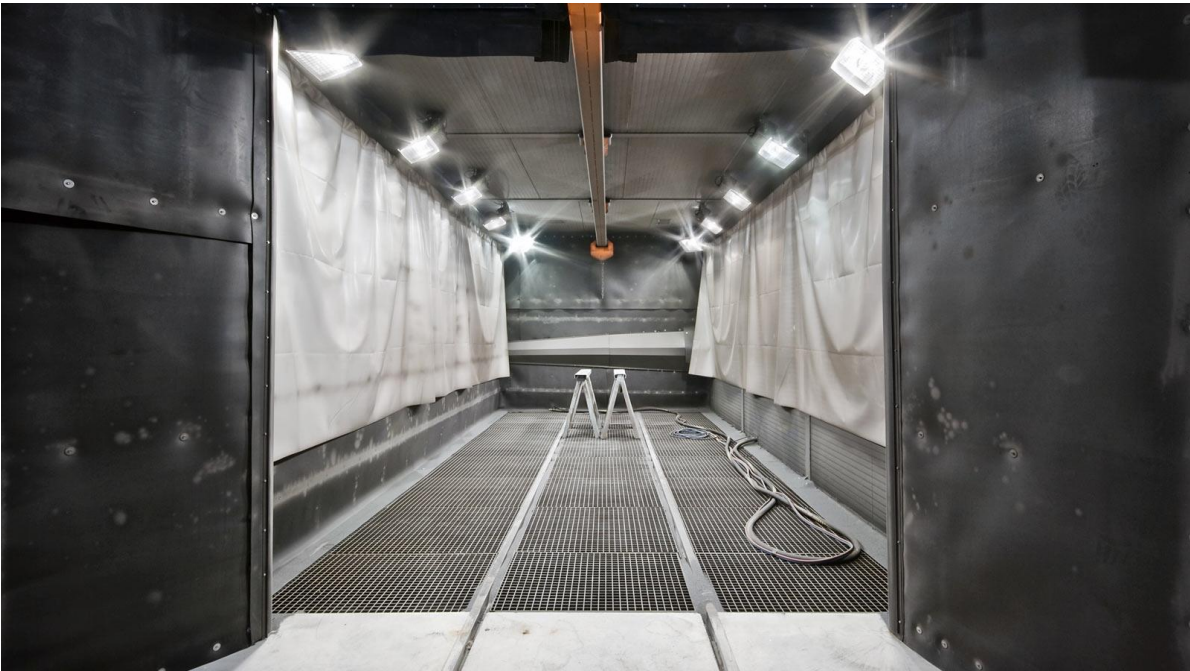
Blasting room 10x5 metres with carrier trolley and overhead C track (up to 300kg), scraper floor recovery system.
