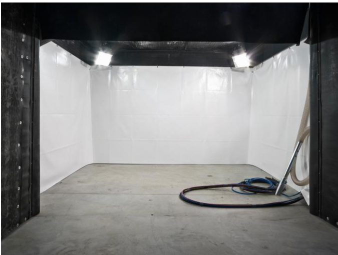
Blasting room interior with pneumatic suction.
